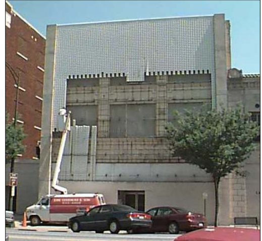
The removal of false façades is encouraged
