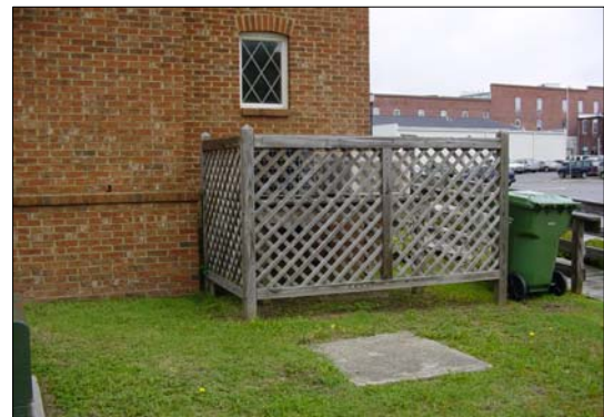
Mechanical systems should be screened from view.
