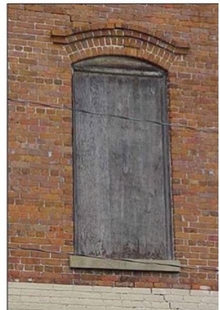
Closing in window opening with masonry or plywood is not appropriate
