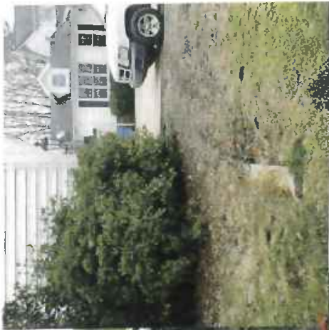
Damaged junction box receives drainage from Larkhaven Lane and Melchor Road 30" and 15" pipes combine with 18" outflow
