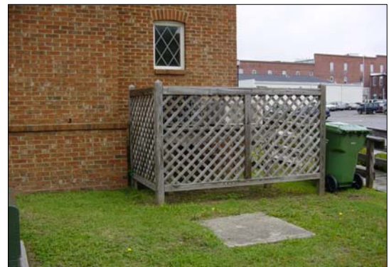
Mechanical systems should be screened from view.
